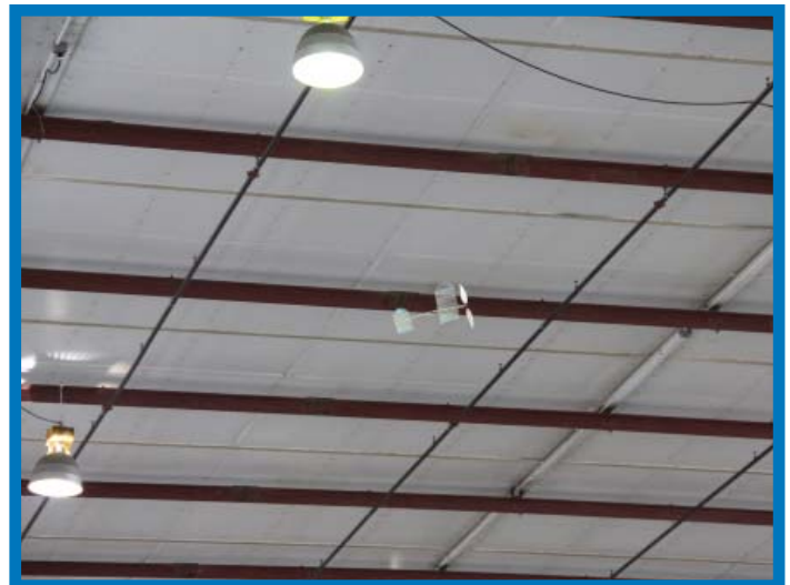
One of the Team Layne models up near the ceiling. Note the curved propeller tips.
